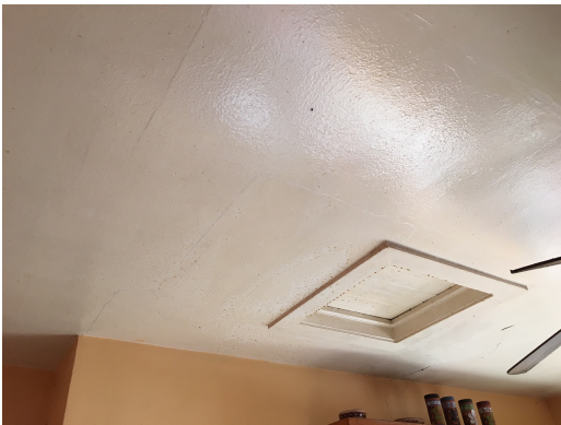
Dillard Ranch - House - Kitchen Ceiling
