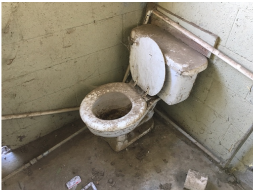
Dillard Ranch - Outbuilding Shed - Toilet
