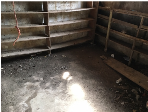
Dillard Ranch - Well Pump - Basement Floor
