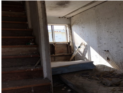
Dillard Ranch - Well Pump - First Floor Room
