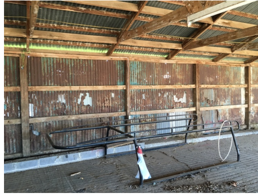
Dillard Ranch - Outbuilding Shed - Rusted Walls
