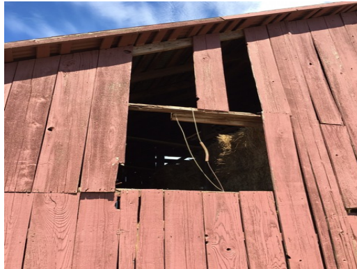
Dillard Ranch - Barn2 - Missing Panels
