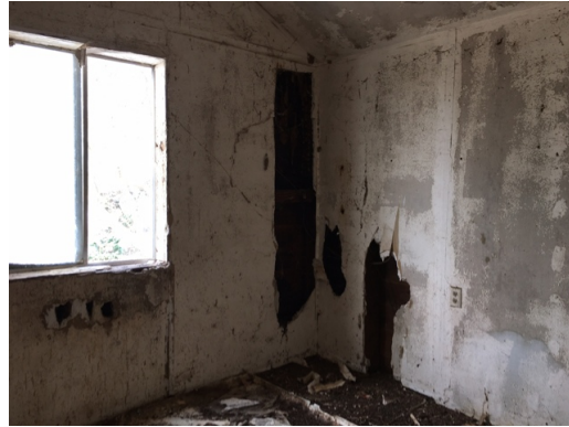
Dillard Ranch - Well Pump - Second Floor Interior
