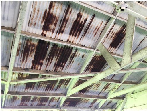
Dillard Ranch - Outbuilding Shed - Rusted Roof
