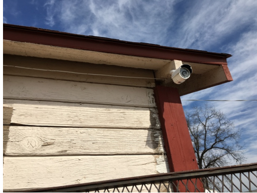
Dillard Ranch - Outbuilding2 - Security Camera
