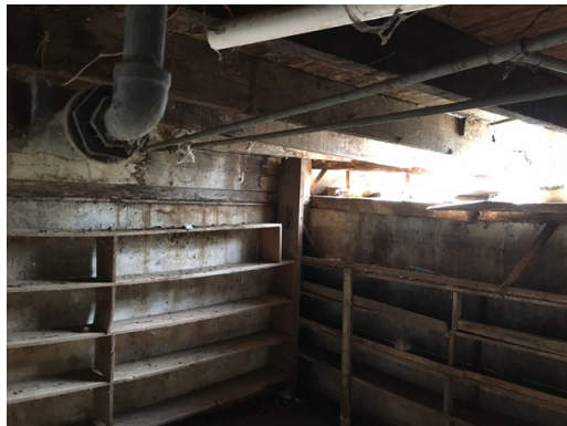
Dillard Ranch - Well Pump - Basement
