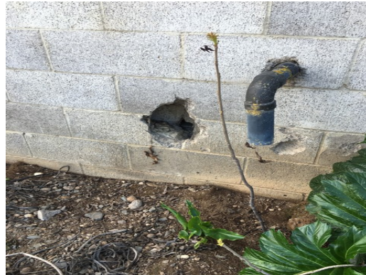
Dillard Ranch - Outbuilding Shed - Exterior Wall Damage
