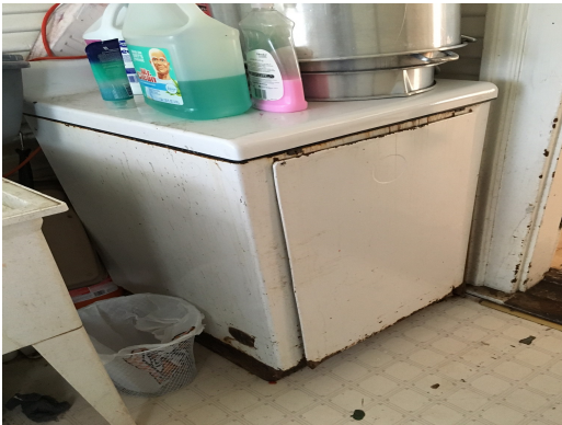
Dillard Ranch - House - Water Heater
