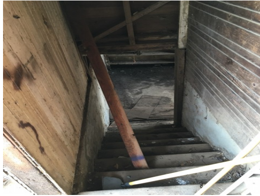
Dillard Ranch - Well Pump - Basement Stairs
