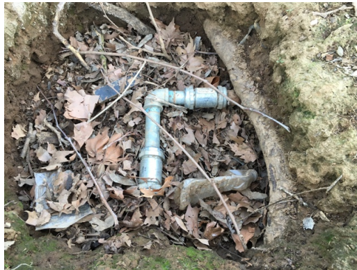
Dillard Ranch - House - Domestic Water Piping
