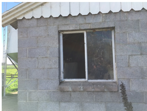
Dillard Ranch - Outbuilding Shed - Missing Window
