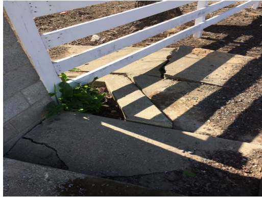
Dillard Ranch - Outbuilding Shed - Concrete Path Damage
