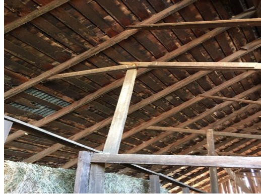
Dillard Ranch - Barn1 - Broken Roof Support
