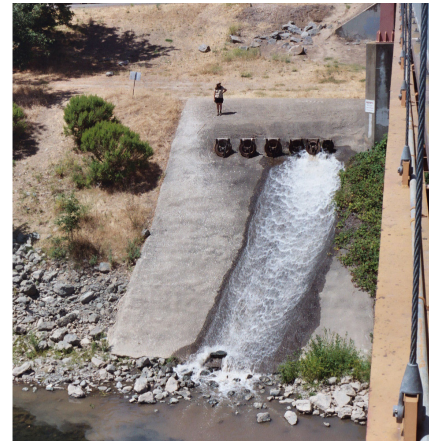
An outfall emptying runoff from the California State University, Sacramento campus into the LAR channel in the Campus Commons Area. Photo Credit: Regional Parks
