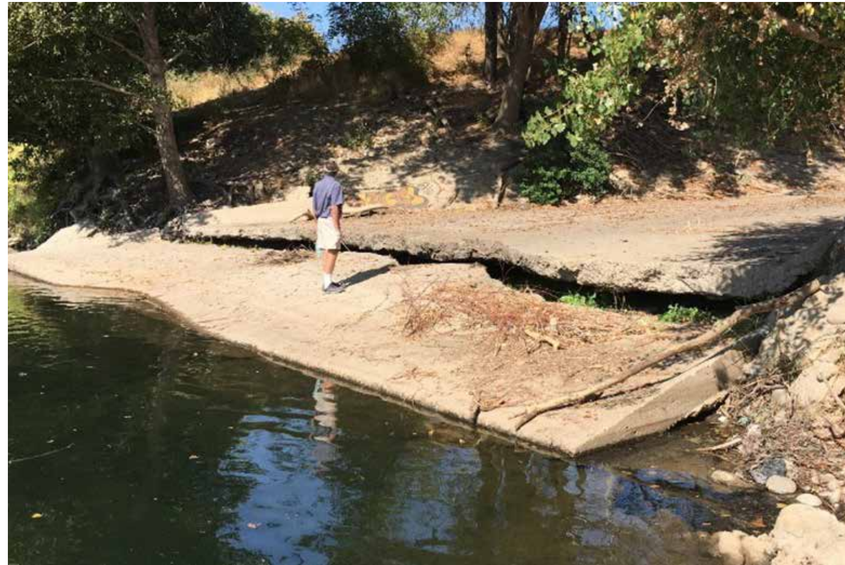
FIGURE 5-13 LARGE URBAN STORMWATER OUTFALL WITH BROKEN APRON (~RM 5.3)
